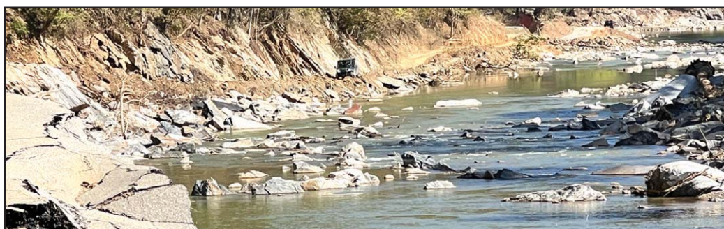
The roadway leading into the Little Creek Community has been 'rebuilt' to a small one-lane dirt and gravel lane sitting precariously on the riverbank of the Cane River.
