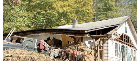
Damaged homes and vehicles can be found throughout every community.
