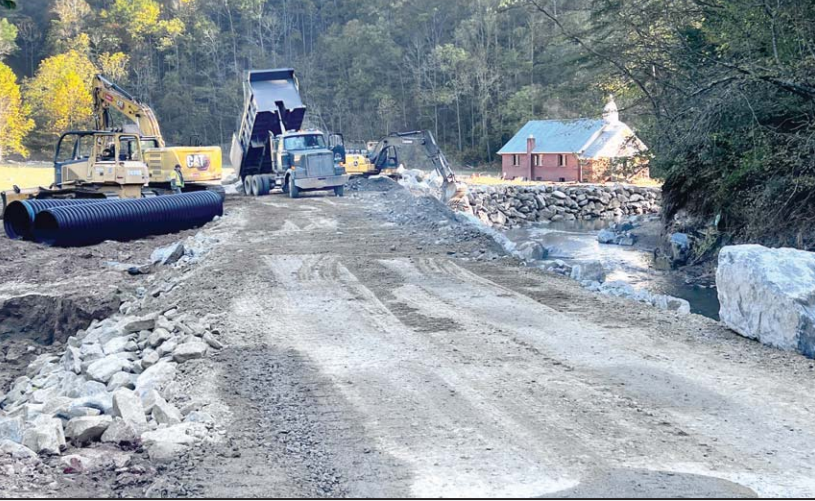
The damage to roadways due to Helene is immense. Flooding not only took the pavement, but the roadbed underneath. Repairs have begun, but many will remain with one-lane access for many days to come.
