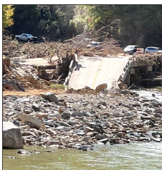
Communities have been cut off due to the destruction of bridges and roadways.
