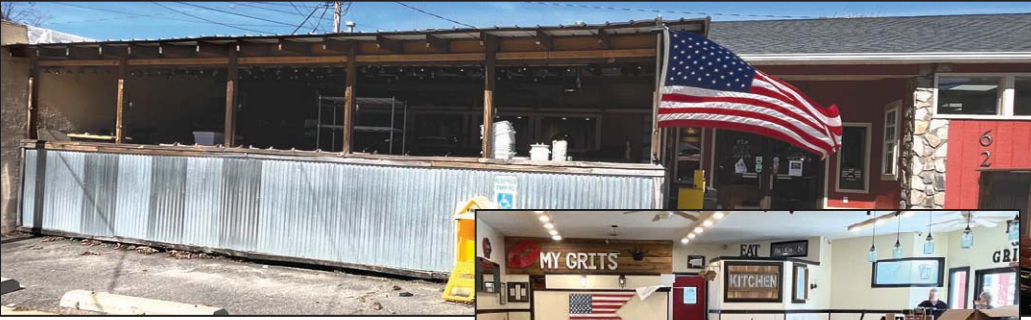
Leigh Howell, owner of Pig n Grits restaurant in Burnsville, has suffered water damage. They are working tirelessly to get those damages repaired. They hope to be able to open back up soon and look forward to seeing their loyal customers.
