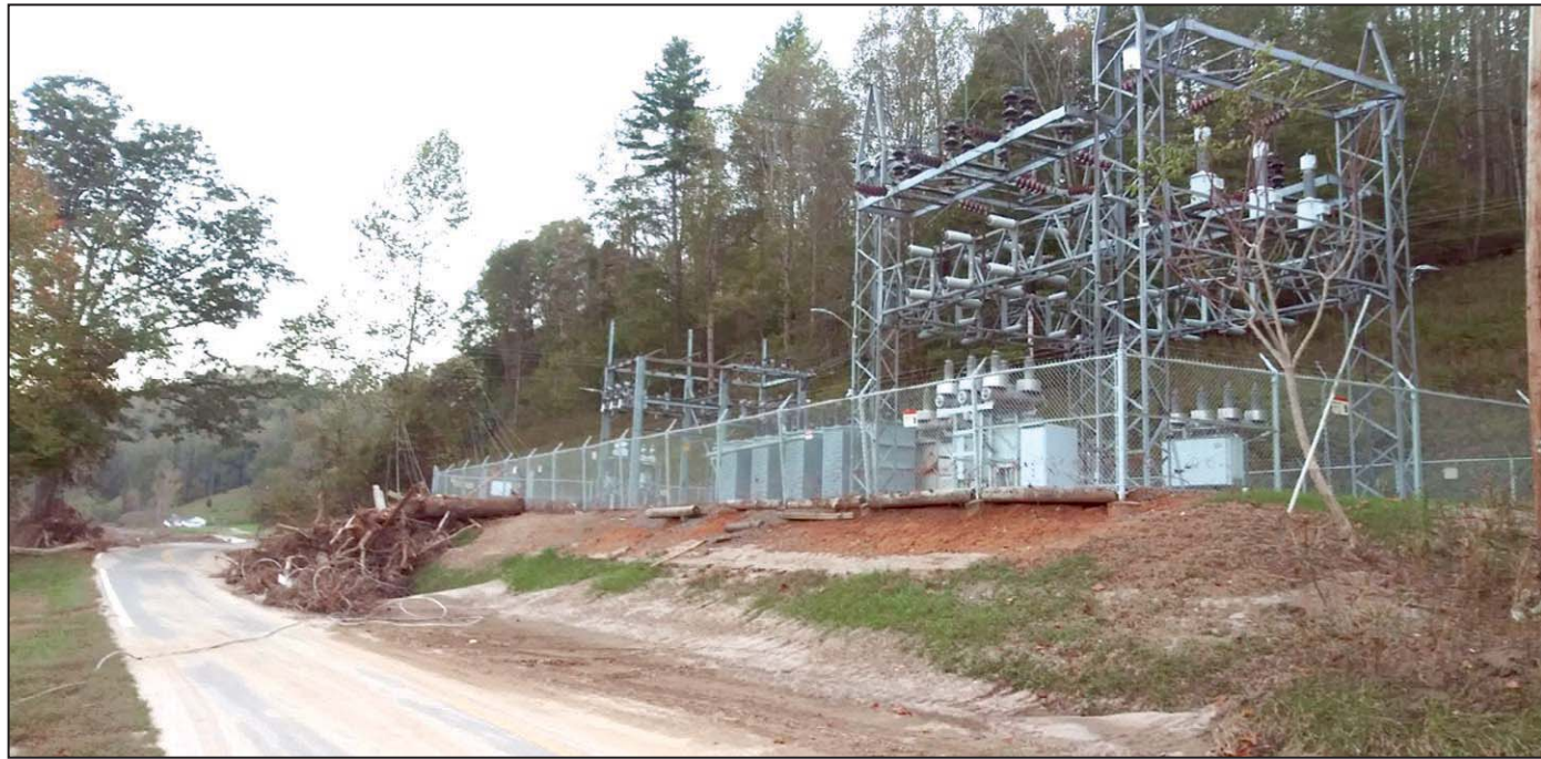
The Relief Substation was one of the areas hit by high water from the Toe River
