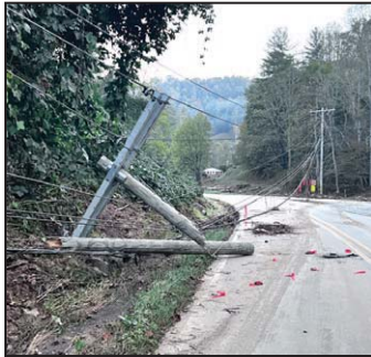
Broken poles and downed power lines throughout Yancey County have proven an obstacle for restoration of service.
