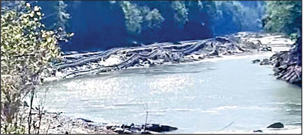
Damage from Helene has turned one section of the Blue Ridge Subdivision of the CSX Corp. rail line in the Poplar Community of Mitchell County into what appears to be more suitable for a roller coaster ride over a commercial train.
